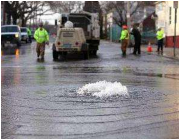
TARIQ ZEHAWI/STAFF PHOTOGRAPHER A December water main break in Passaic flooded roads and disrupted water service for residents.
